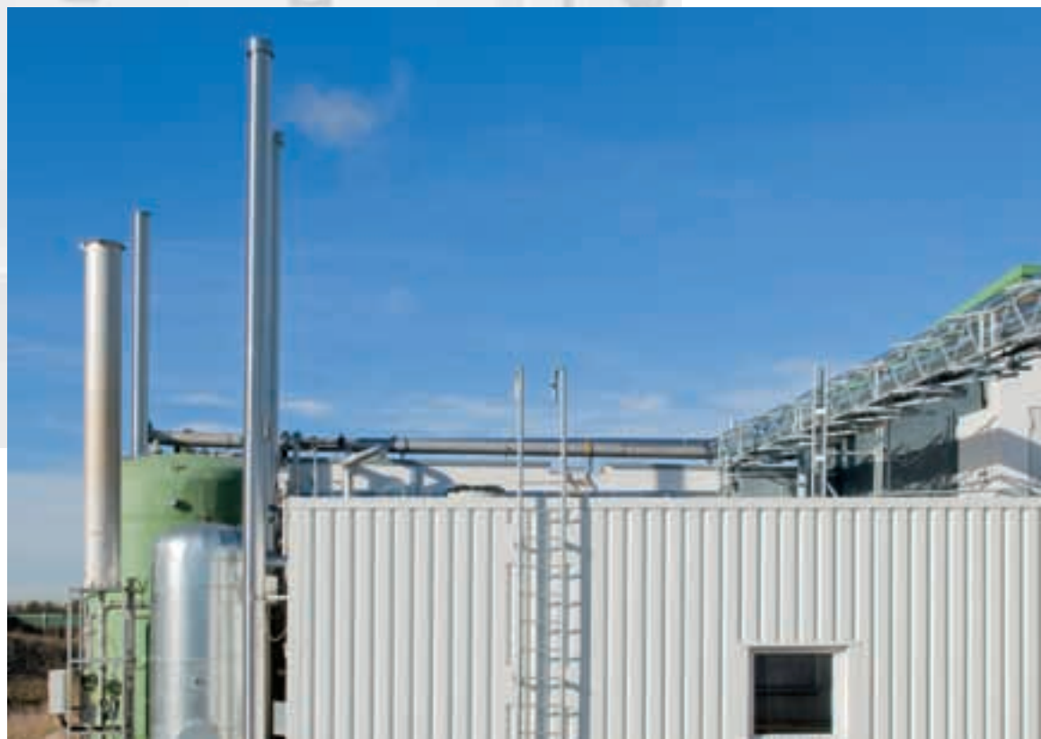
Combined heat and power plants (CHP)
